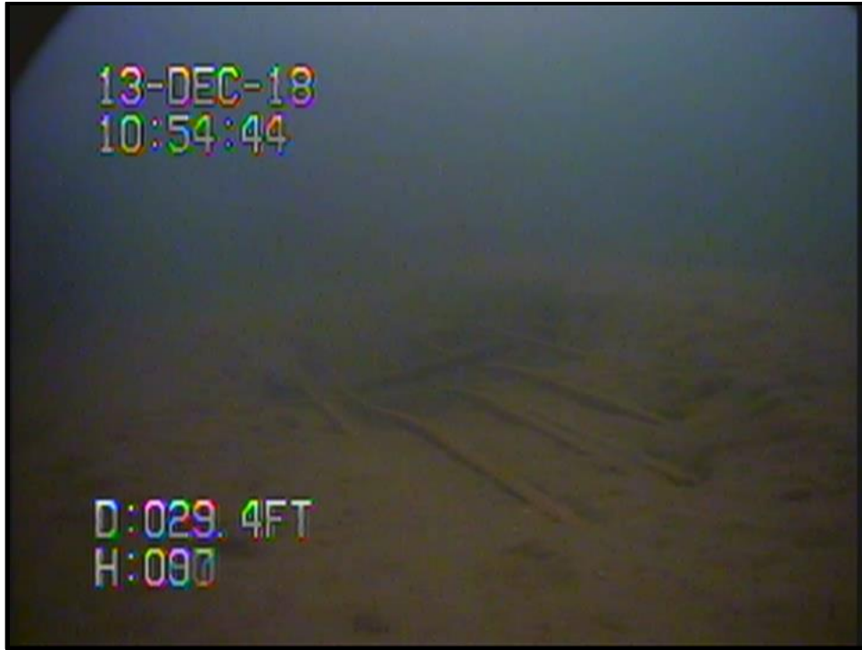
Figure 10 Typical apron erosion damage found downstream and between baffle block rows.
