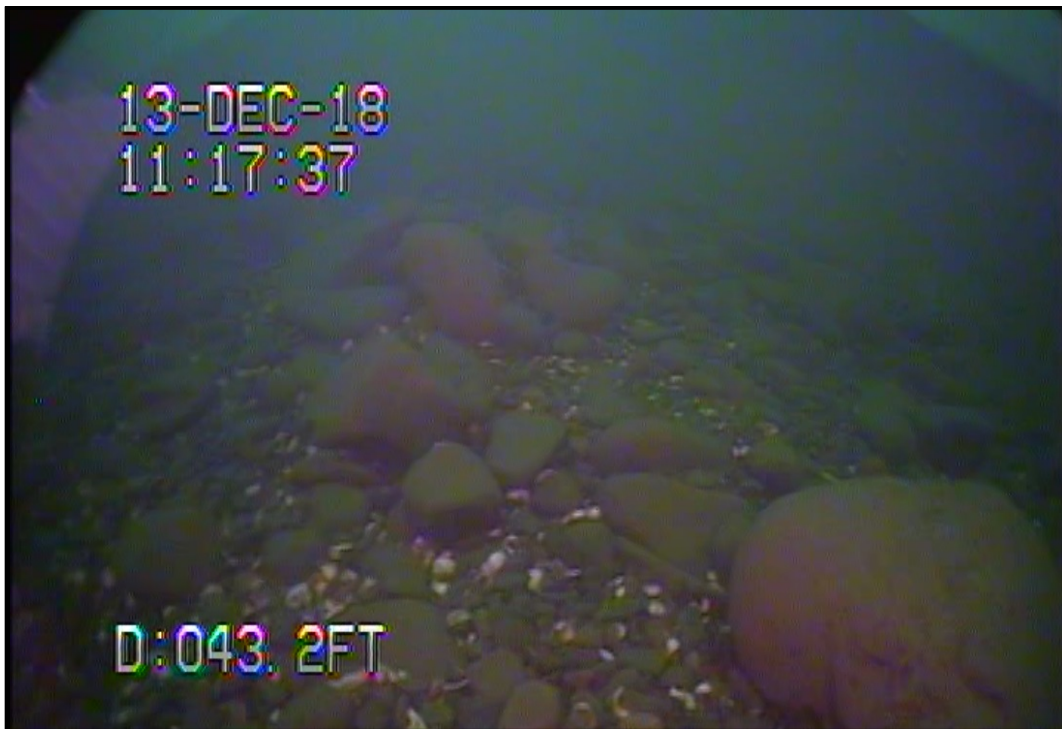
Figure 7 Another image of rock below SB 10-12 End Sill.
